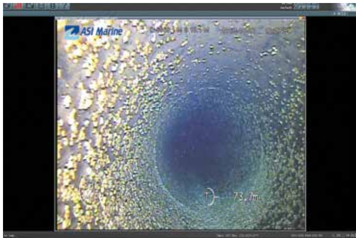
Figure 1. ROV pictures showing quagga mussel build up prior to pigging
