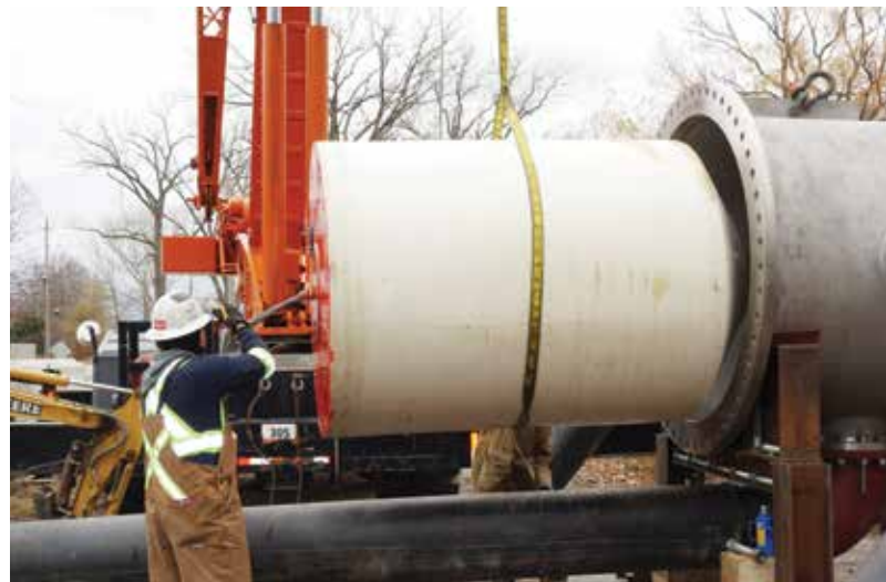
Figure 3.60-inch durafoam style pig being placed in launcher
